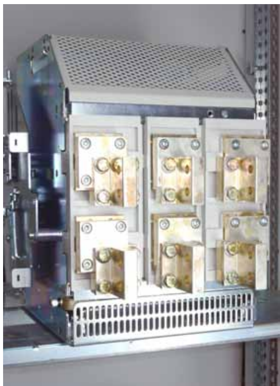
Draw-out DMX 3 size 1, 3-pole, equipped with retrofitting kit, with reuse of DMX orientable connectors
