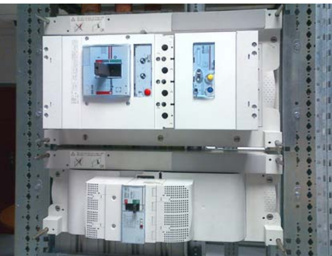
DPX and DPX 3 circuit breakers are mounted horizontally on the bases.
